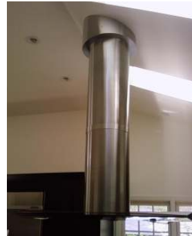
Stainless Steel Duct Surround
